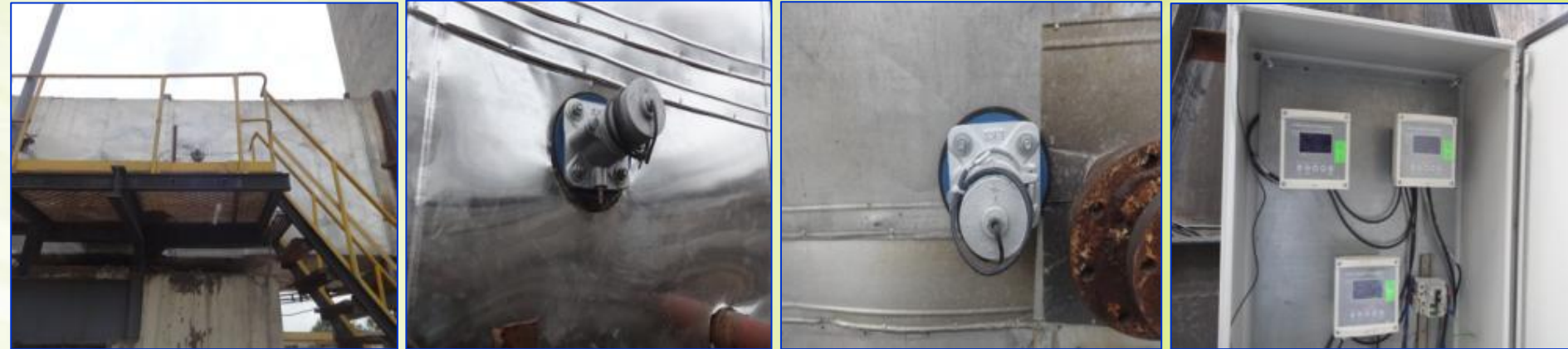
Installed Transmitter & Receiver on Boiler Duct and Local Display
