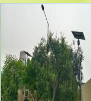
Solar Unit at Plant
